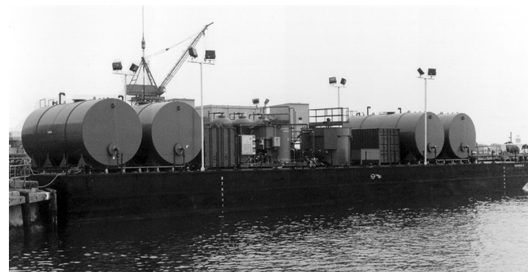
The TBT treatment plant resides on a barge that can be moved between dry docks as needed.
