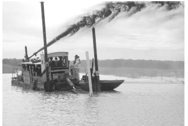
Spray dredging is a version of hydraulic dredging. Underwater sediments are cut loose by a rotating head on the dredge. The sediment is mixed with surrounding water and sucked into the dredge by a powerful pump. The slurry is then forced, under great pressure, through a hose and nozzle, which can spray the mix up to 100 feet over adjacent areas.
