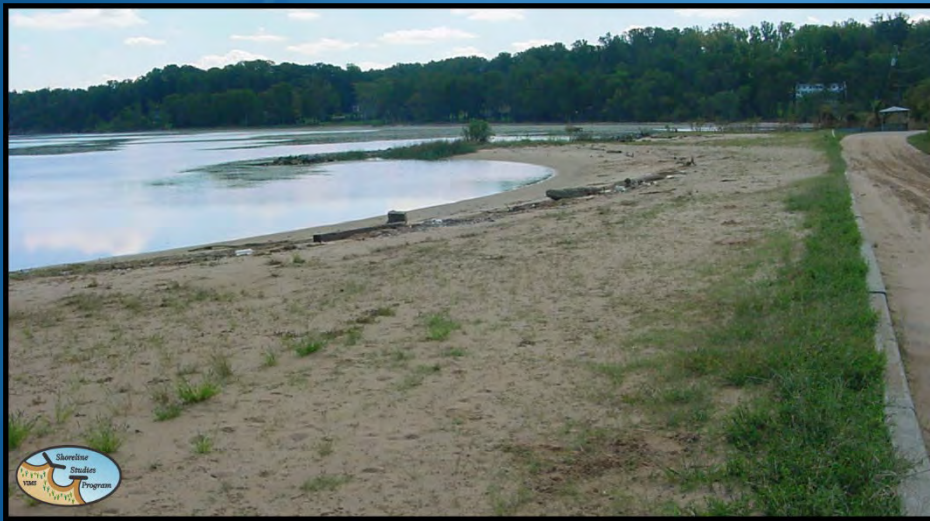
Aqua Landing shoreline on 30 September 2003 post Hurricane Isabel. Though sand washed over the jersey wall, overall the system is intact
